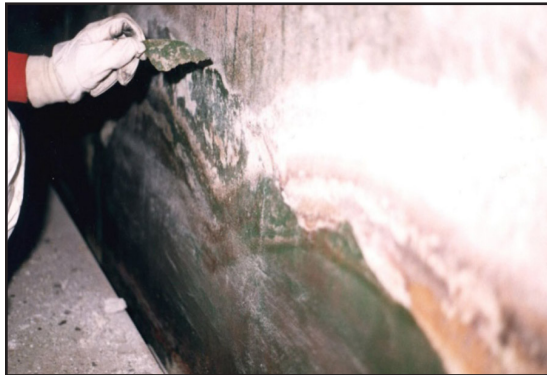
Glass flake reinforced vinyl ester coating delaminating from substrate after <2 years in service
